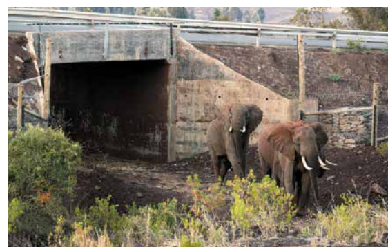
Figura 39: Box culvert en Kenia, para paso de elefantes. Fuente: (Straziuso, 2011). Tomado de Internet: https://tucson.com/news/science/environment/kenya-elephant-underpass-a-hit/article_fe50f43e-b5a4-5134-a353-8c3fab6496cf.html
